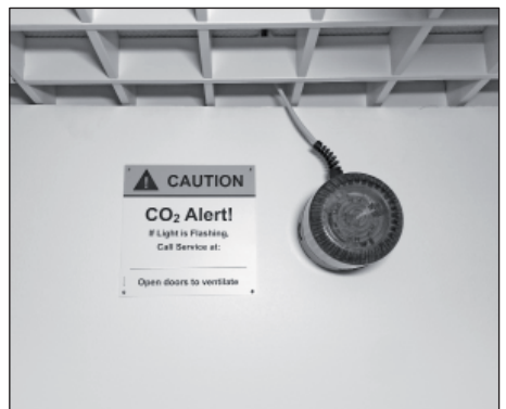
Warning lamp with sign
