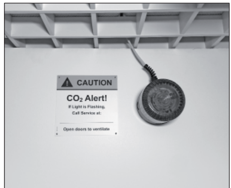
Warning lamp with sign
